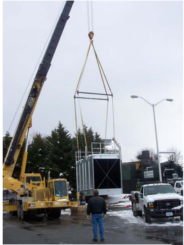
Cooling Tower at Wallace Hall
