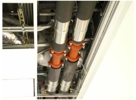
Condenser Water Piping
