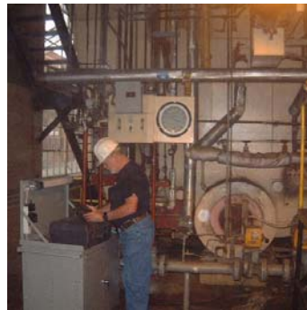
Calibration of Boilers
