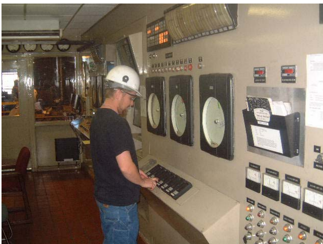
Boiler No. 7 Controls
