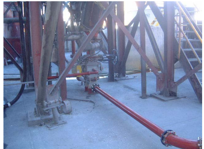
New Waste Lime Conveying System
