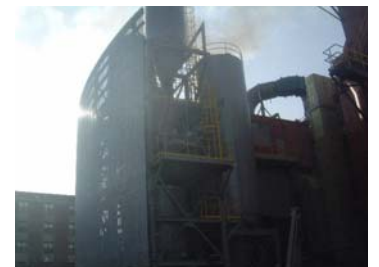
New Air Pollution Control System
