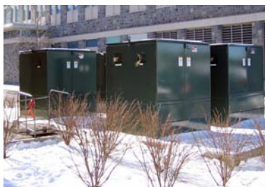
New Transfer Switches at Derring Hall
