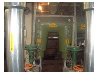
Steam Pressure Reducing Station
