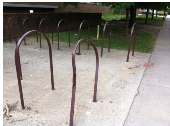
Damaged Staple Racks in the Upper Quad
