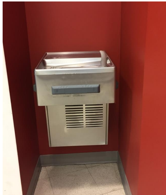
Water Fountain in 5 th floor: Next to the elevator door
