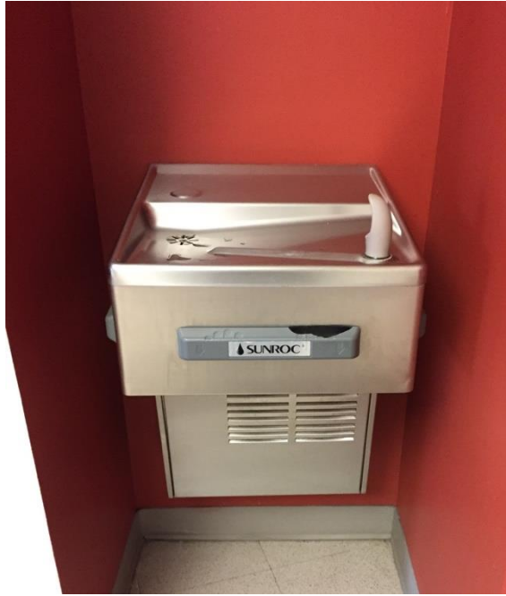
Water Fountain in 4 th floor: Next to the elevator door
