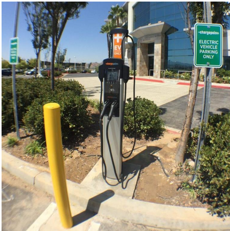
Figure 1: A ChargePoint EV charging station. [Source: https://signalscv.com/2019/11/city-installs-additional-electric-vehicle-charging-stations/ ]
